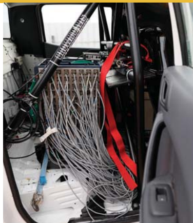
ABOVE: Design of the Ranger’s cab. LEFT: Wiring systems in contemporary vehicles require a team with a diverse range of skills.
