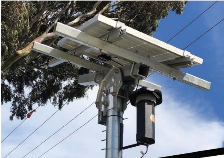
LEFT: SiteHive Hexanode on a solar panel. BELOW: SiteHive cloud software provides access to live site data.
