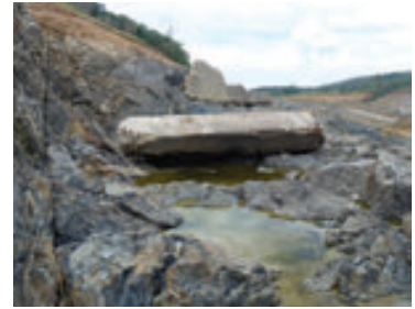
RIGHT: Damage from the 2013 flood included scouring and erosion downstream.
