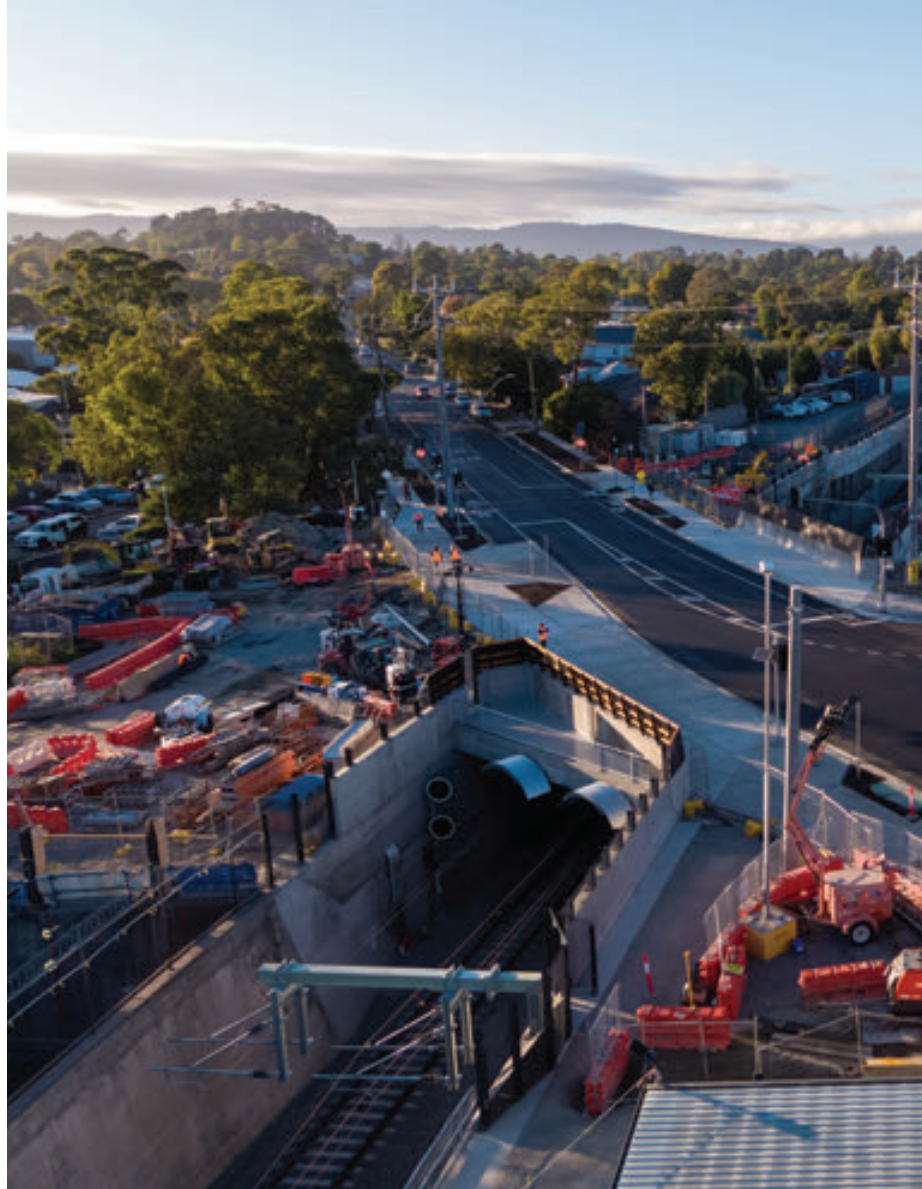
RIGHT: A new rail trench has replaced the level crossing at Bedford Road in Ringwood, northeast of the Melbourne CBD.
