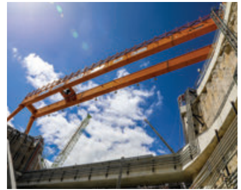
RIGHT: The largest registered jack-up barge in Australia, installing the intake structures; the view from within the Alkimos facility.
